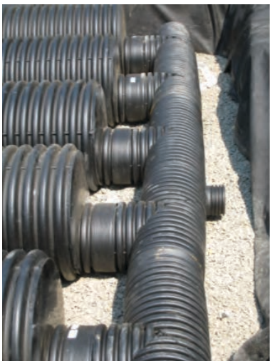
Welded reducers used in a storm water detention application
