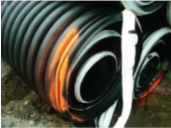
Damaged pipe, marked and set aside.
