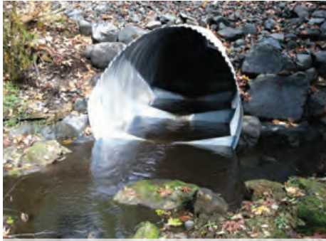
BEVELED END with WEIRS: The addition of notched, log or straight rock retention weirs are beneficial to adding an additional controlling feature to any culvert. These are an ideal addition when the need to control fish passage is present.
