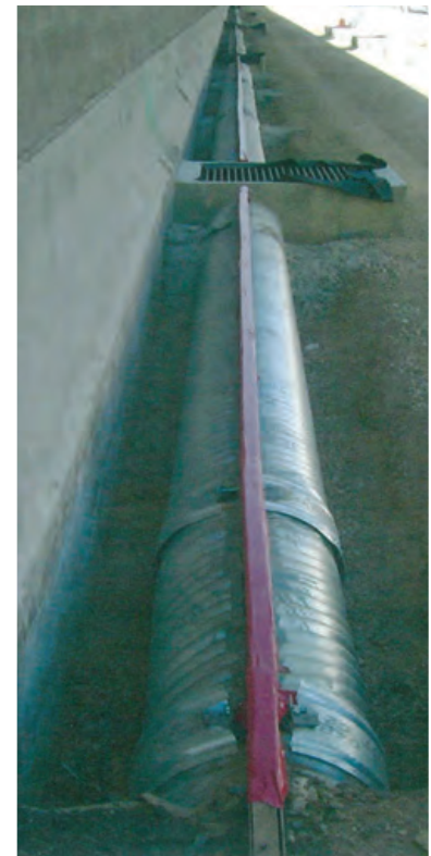
COVER TOP OF GRATE WITH TAPE OR OTHER MATERIAL TO KEEP GROUT AND PAVING MATERIALS OUT OF PIPE.
